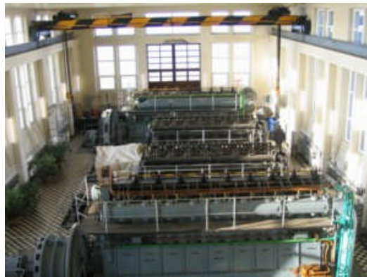
View at the generator room Radio Luxembourg Photo: Hans Knot
